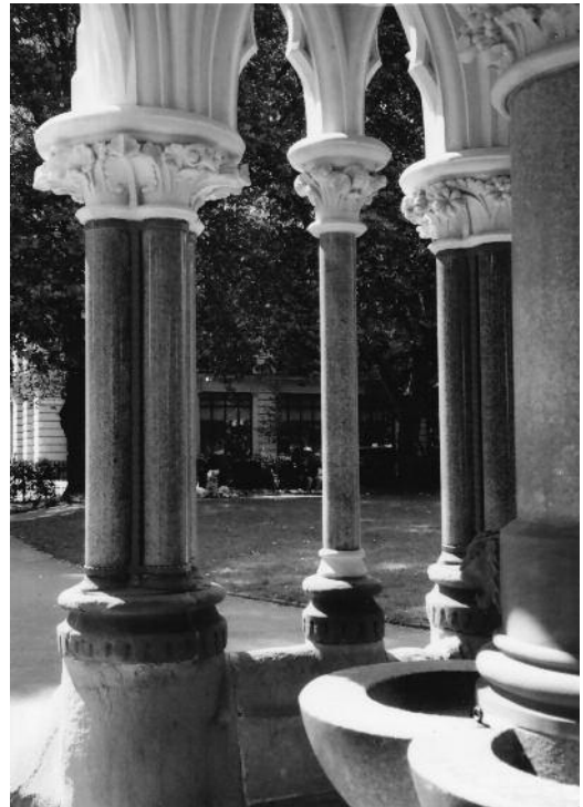
Frost-damage to the Pennant Sandstone (ER)
